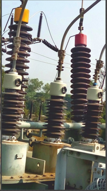
52 kV OIP bushing as Retrofit to damaged OIP Bushing at MPPTCL
