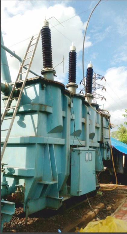
145 kV OIP bushing as Retrofit to old 145 kV SRBP Bushing at MPPTCL Khandwa
