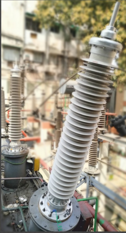
145 kV RIS bushing as Retrofit to old 145 kV OIP Bushing at CESC
